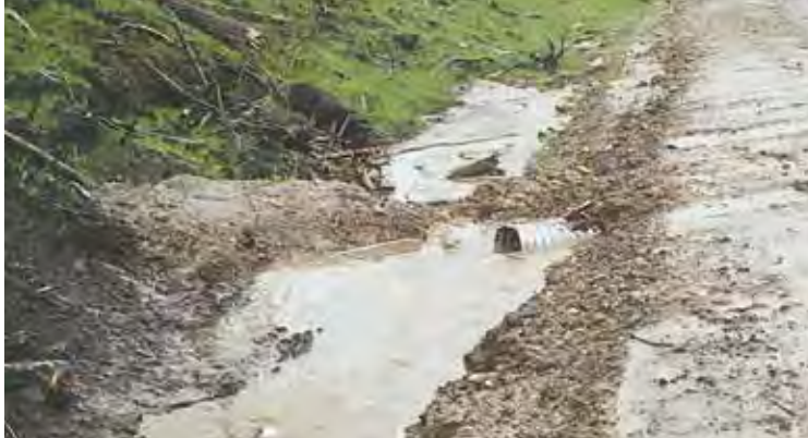
This undersized cross-drain culvert resulted in a breached ditch block and sediment flowing directly into the stream. With proper cross-drains, water cannot soak into the road, causing surface softening and rutting.
