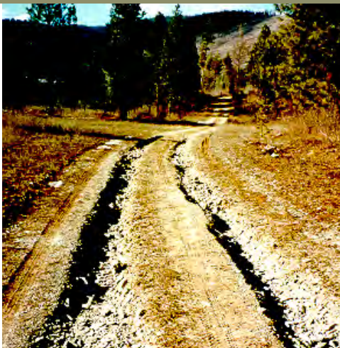
Water runoff formed these long narrow chutes or rills, running down-slope on the surface of this road. It is a source of sediment.
