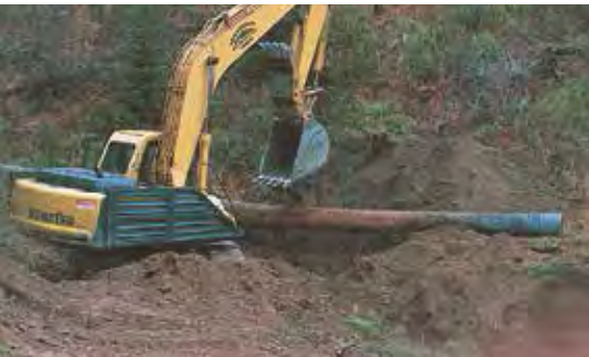
Removing culverts can prevent erosion problems, and water bars may be a solution. Space water bars more closely in areas likely to erode. Cut and fill slopes may need to be extended to a more natural grade.
