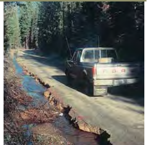
This plugged cross-drain culvert and washed-out catch basin can be a source of sediment.
