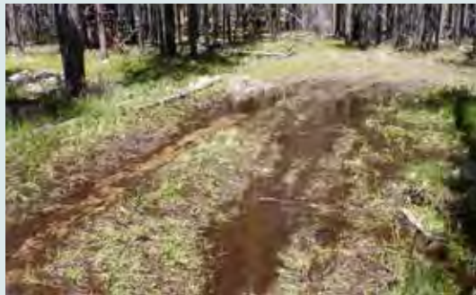
Damage to roads and streams can result from poor crossings and lead not only to washed out roads but to heavy stream sediment loads and damage to streams and fisheries.
