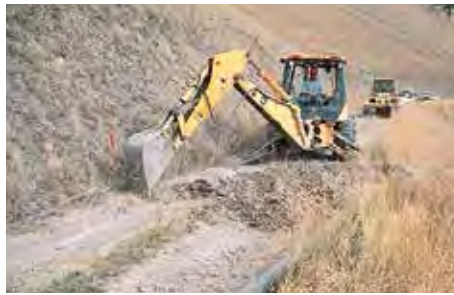
A backhoe is the best choice for open top pipe culvert installation.
