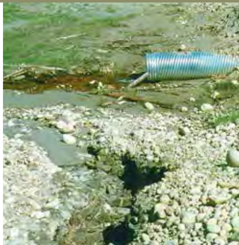
This ditch flowing directly into a stream has resulted in sediment delivery. An additional drain culvert or rolling dip should be installed.
